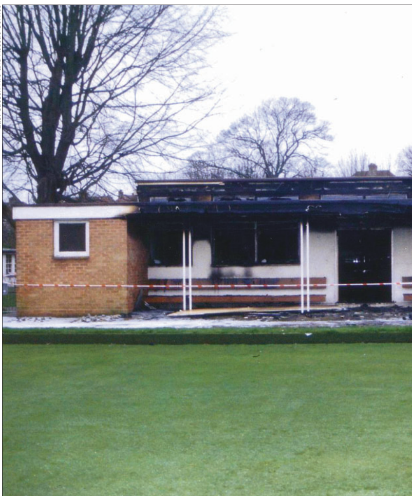
Investigators believe that the fire that spread through this sports pavilion was started deliberately
